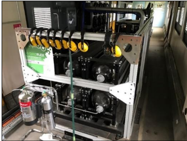
Figure 7: 4x Compressed Hydrogen Storage Tanks Inside HydroFLEX 1 (courtesy of VSTS)
