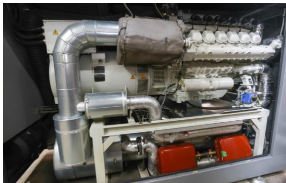
Figure 1: Combined Heat and Power plant in a hospital in Coyhaique in the south of Chile
