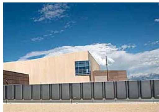
Figura 28: Fuel Cells en eBay Inc. Salt Lake City, Utah, EE.UU [77].
