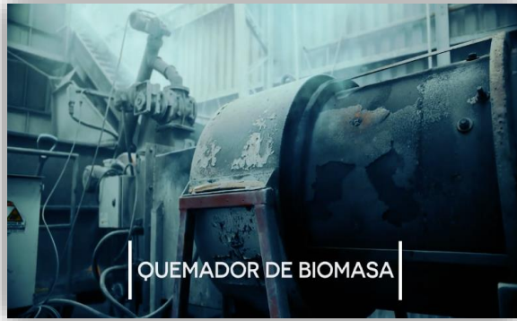
Biomass burner for industrial processes (Toralla)
