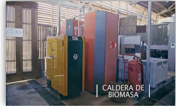
Biomass boiler for the Wine Industry (Viñedos Emiliana)
