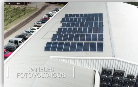
Solar Photovoltaic System in the Agroindustry (Agrícola Hüne)
