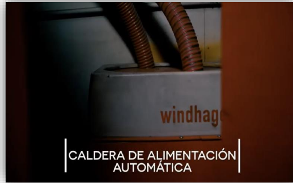
Biomass boiler for the hotel sector (Hotel Vira Vira)
